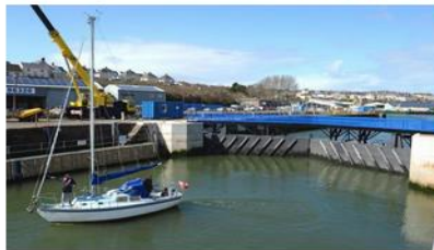
The gates, which weigh 90 tonnes each, were installed as part of a 50m project to speed up lock times and improve accessibility into and out of Milford Docks and Marina.
